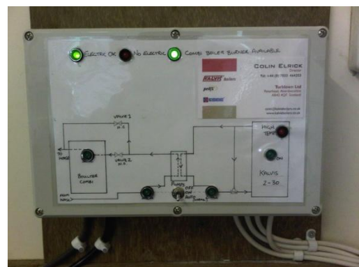
Control panel for automatic changeover of combi and biomass boiler and controlling of backup power supply.
